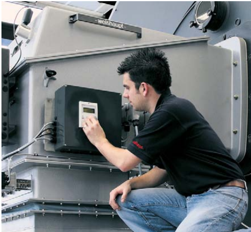
Setting and control of the burner via the ABE display and operating unit
